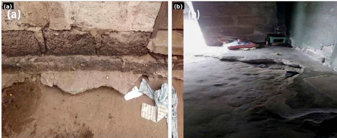
Plate 1: (a) Wall of a residential building affected by flooding at Ganyingbo; (b) Degraded floor of a passage captured at Jofo community (Source: Author, 2018)
